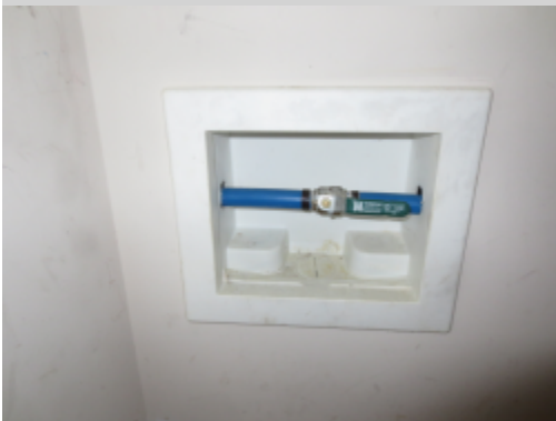
Additional Photograph: This is a photograph of the main water shut off in the front hall closet
