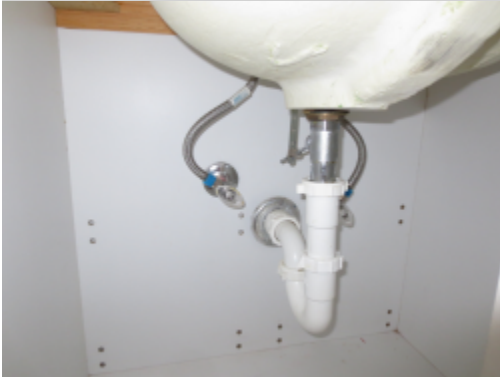
Additional Photograph: This is a photograph of the P trap under the upstairs bathroom sink.
