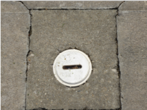
Additional Photograph: This is a photograph of the main waste line clean out in the driveway
