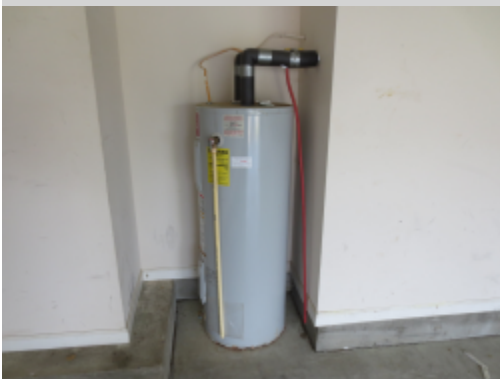
Additional Photograph: This is a photograph of the water heater located in the garage
