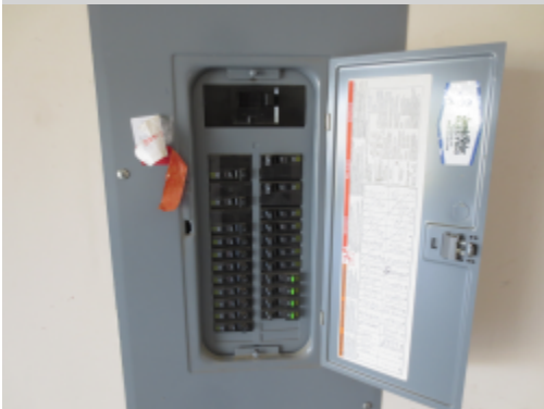
Additional Photograph: This is a photograph of the main electrical panel located in the garage
