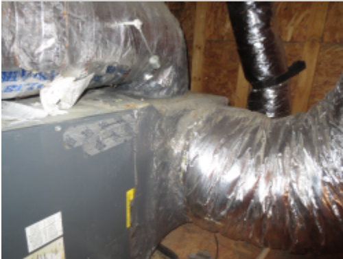
Additional Photograph: This is a photograph of the flexible branch duct work
