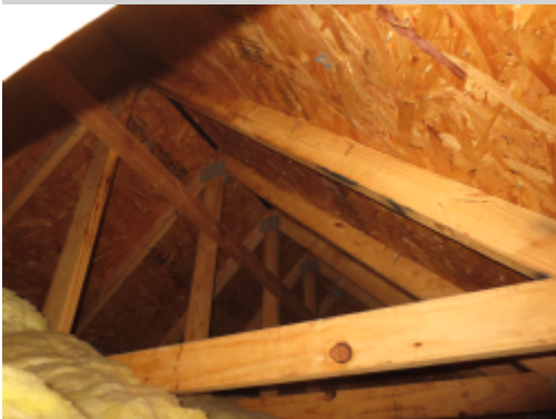
Additional Photograph: This is a photograph of engineered trusses and roof sheathing
