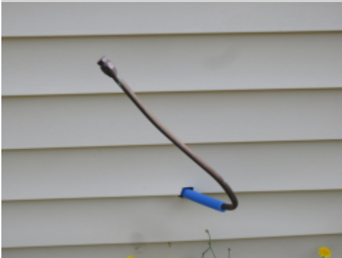
Additional Photograph: This is a photograph of the gas line running to the fire place however there is no fuel tank present
