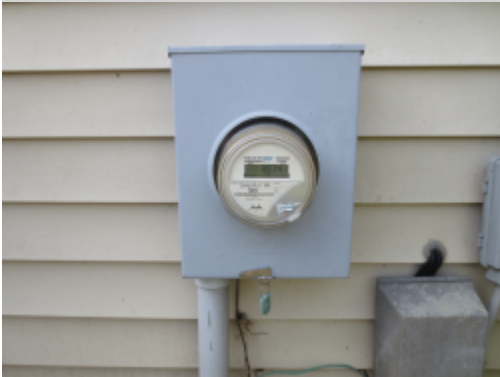
Additional Photograph: This is a photograph of the main service meter located on the left side of the house
