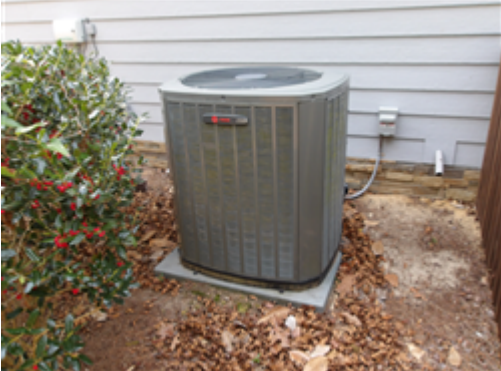
Photo of exterior HVAC unit. This is for your information only.
