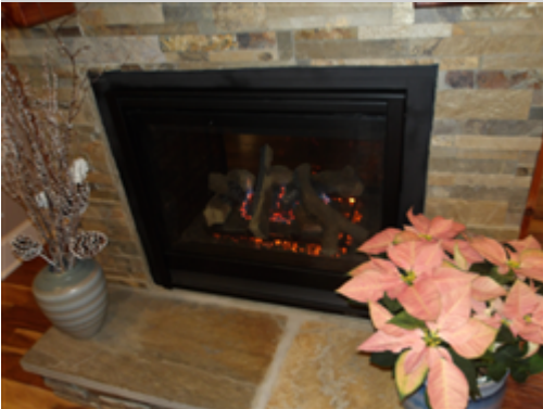
Photo of gas logs in operation. This is for your information only.
