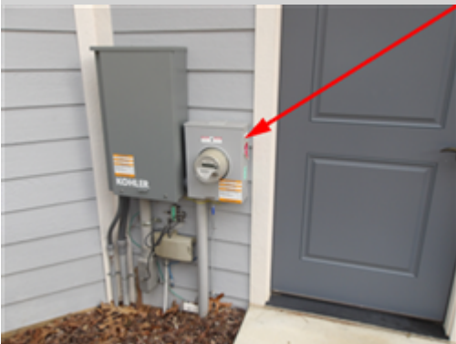
Photo of main electrical service. This is for your information only.
