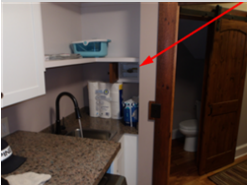
Photo showing emergency water shut off valve located in the laundry room. This is for your information only.
